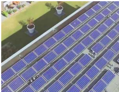
Solar PV ready
